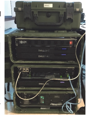
Tactical Server Infrastructure (TSI) Version 2(a) - Large
